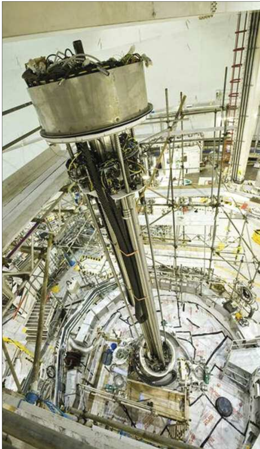
The breeder element removal tool, installed in the DFR's containment sphere. (Photo: DSRL/NDA)
